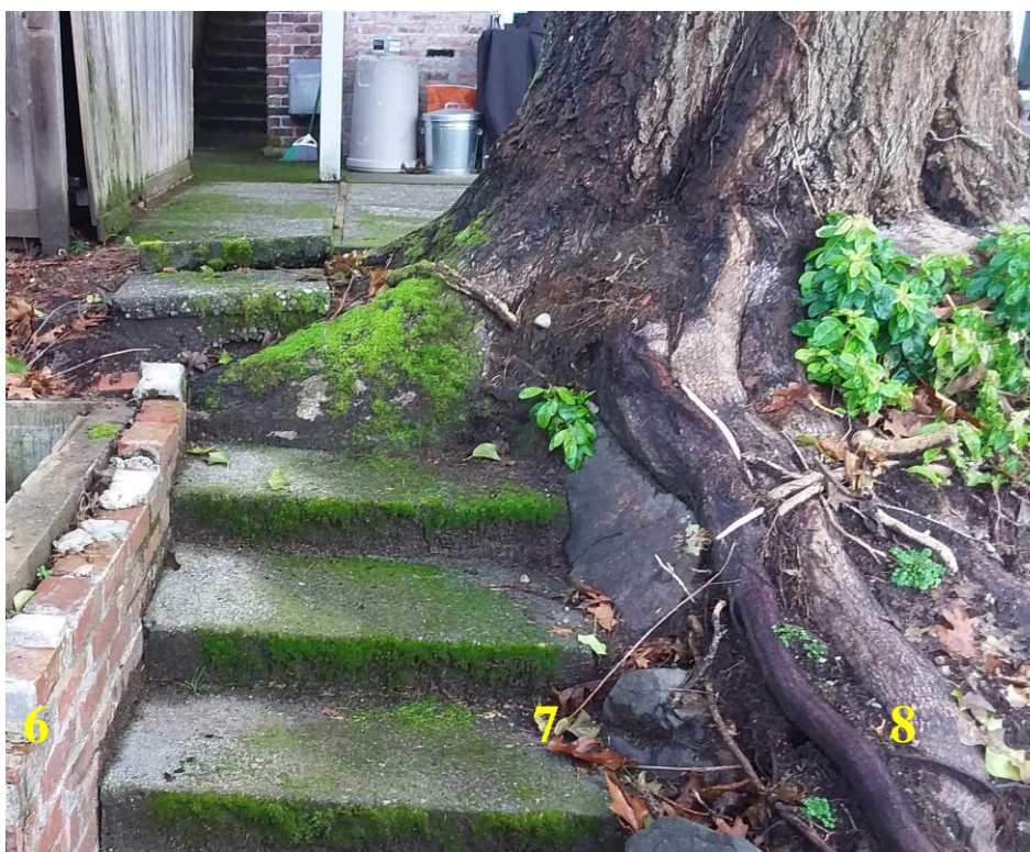
Figure 15. Close up of stairs at the base of the #1 oak.
