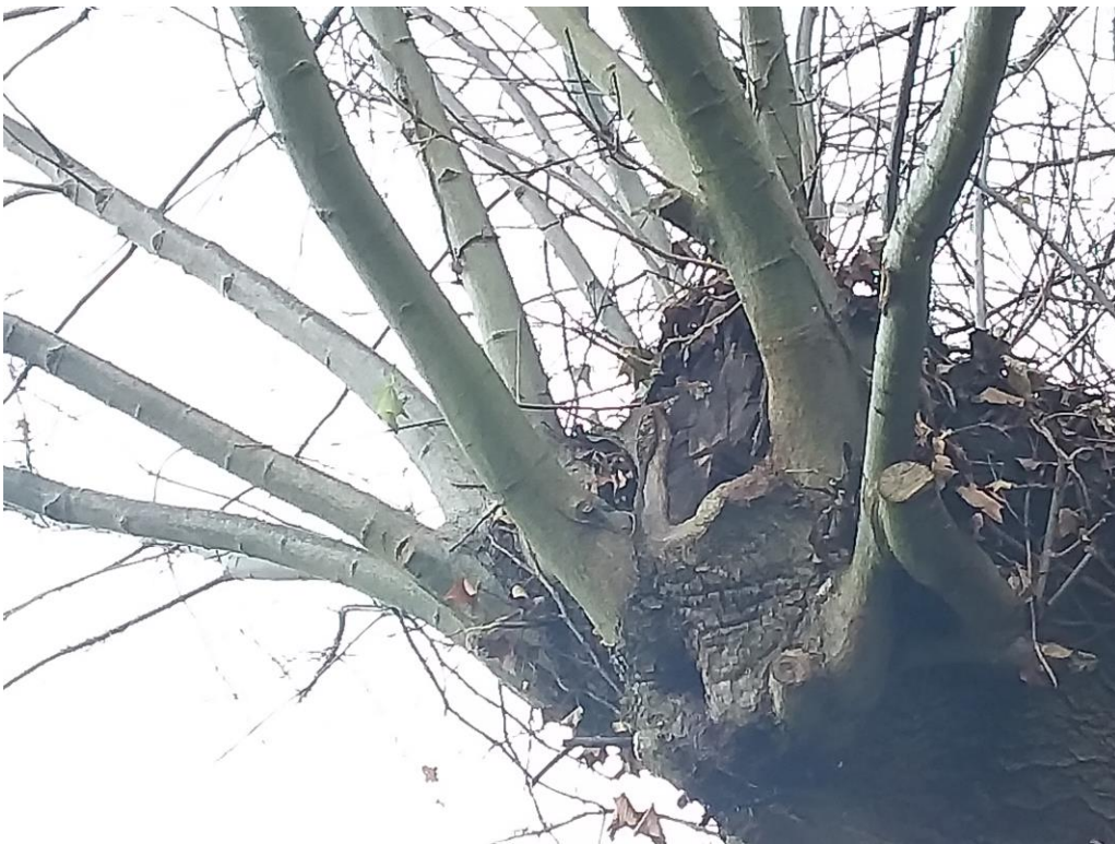
Figure 13. Showing decay and atrophy at another of the stub points on the #1 oak.
