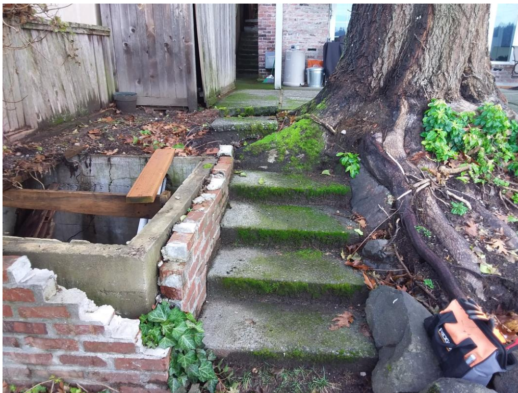
Figure 14. Looking east at the base of the #1 oak showing the pump vault.
