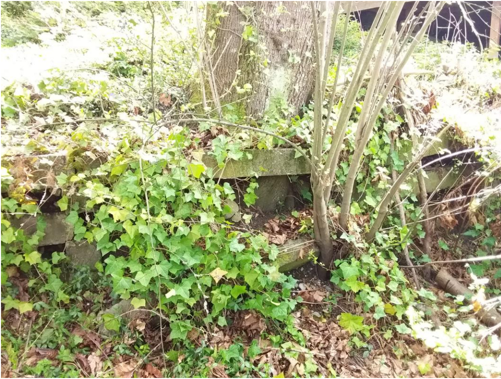
Figure 46. Looking east at the base of the #24 maple coming through the retaining wall.
