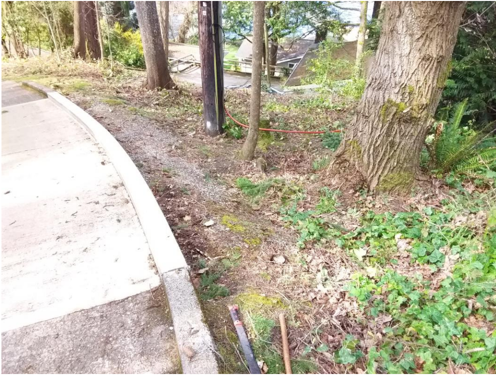
Figure 42. Looking south at the area of new concrete east of the #19 tree.
