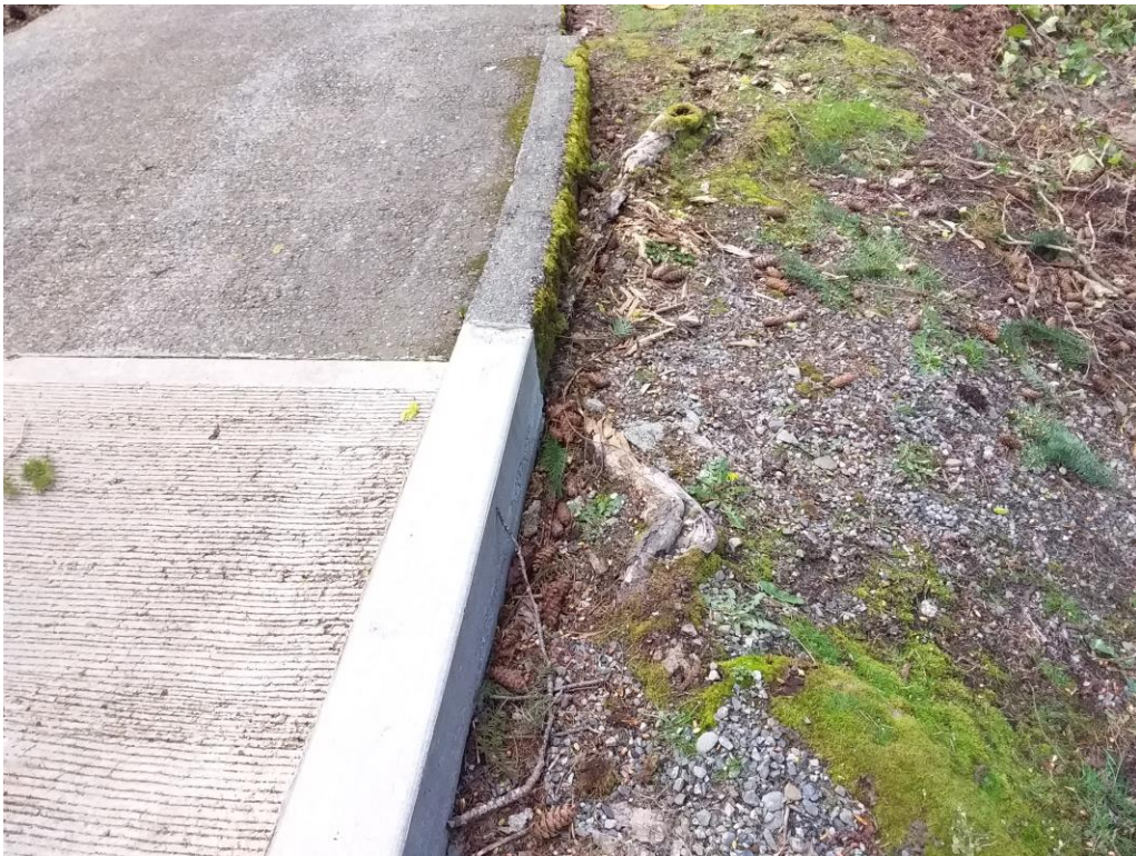
Figure 43. One of the #19 cottonwood roots pushing up against the entry drive curb.
