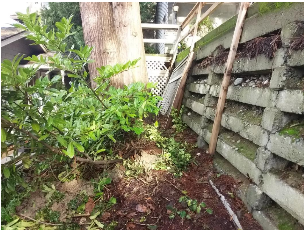
Figure 2. Looking north down the line of the retaining wall system that supports the lower parking area and the garage.
